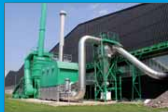
Regenerative Thermische Oxidation
