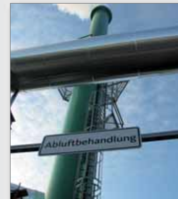
Regenerative Thermische Oxidation
